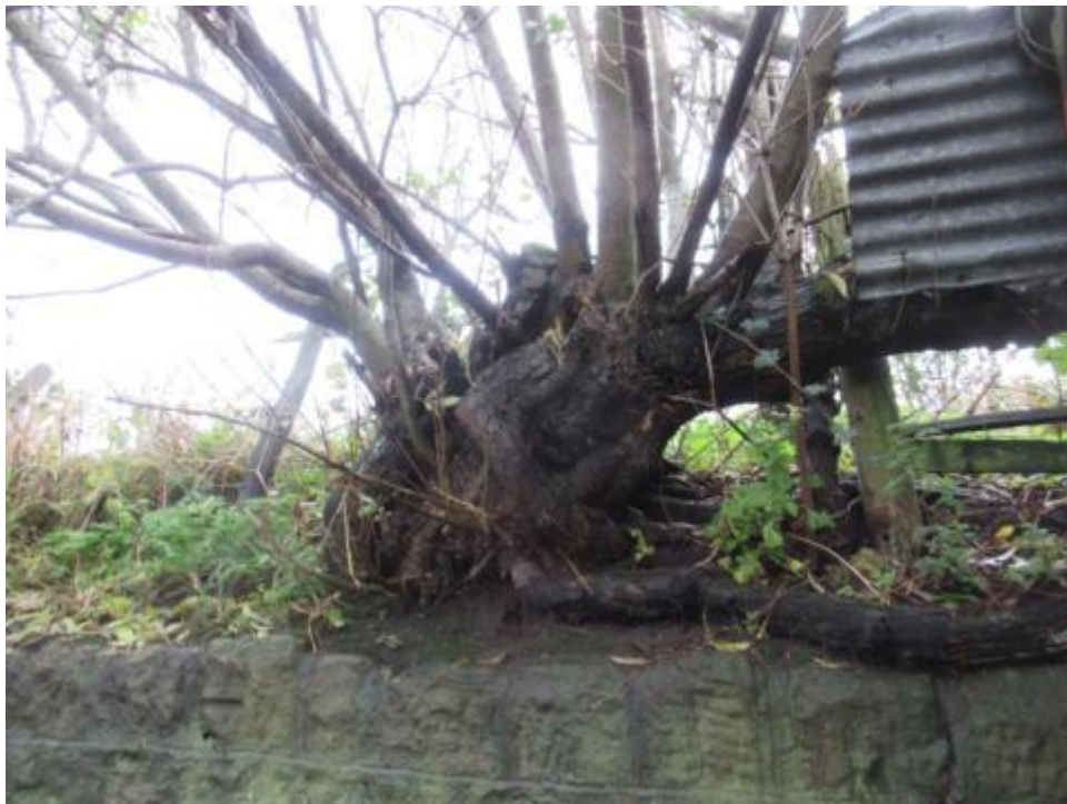
P18 – Tree root growth at the top of the retaining wall
