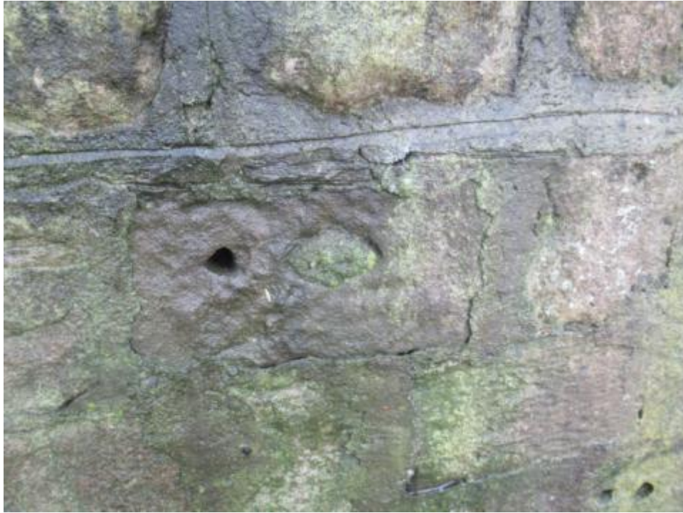
P27 – Hard cement mortar applied to the face of the stone creating ledges, water entrapment and increased erosion of the stone
