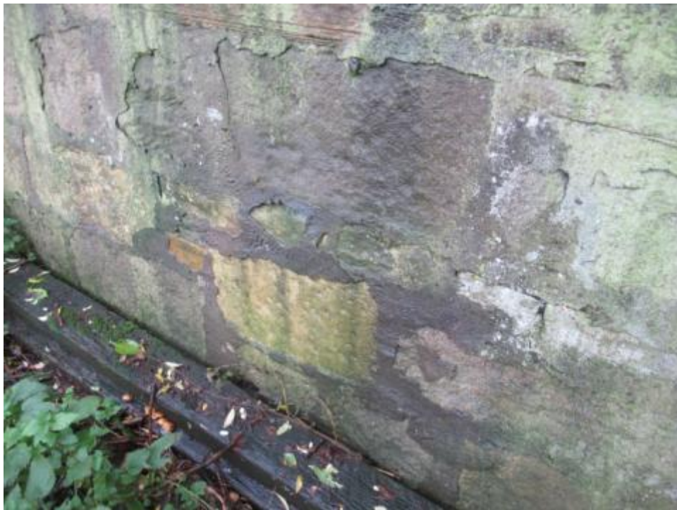
P26 – Hard cement mortar applied to the face of the stone units resulting in increased erosion
