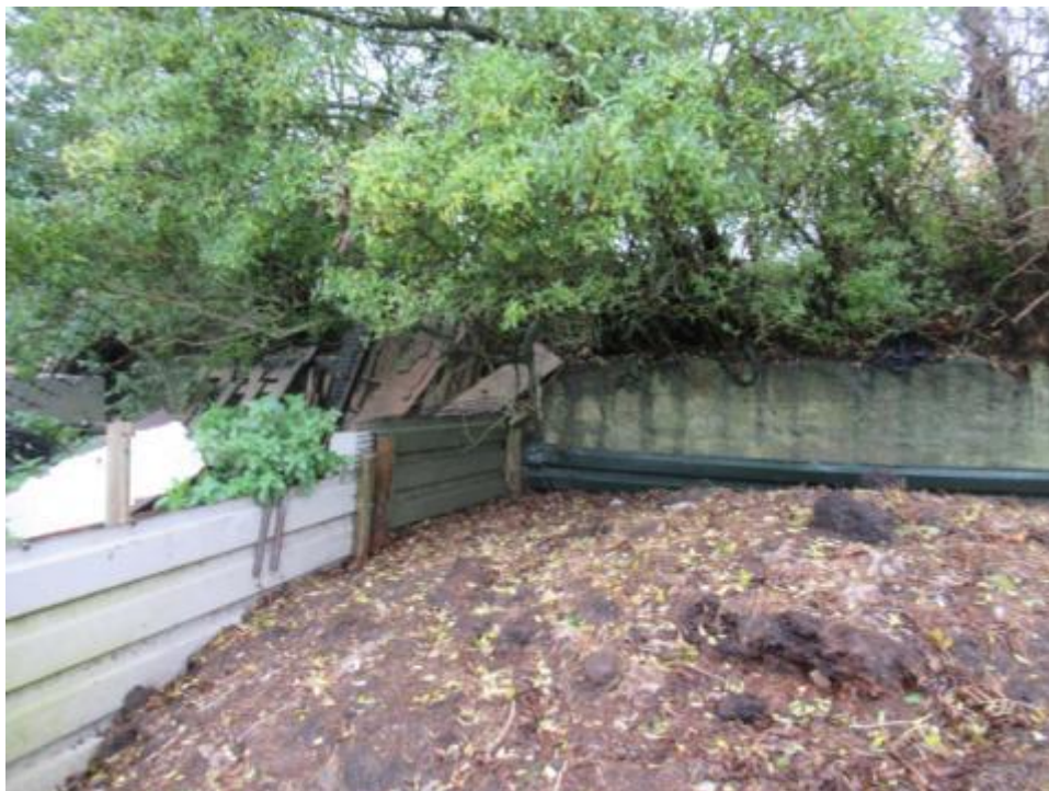
P9 - West Elevation manure heap stacked up against the stone retaining wall
