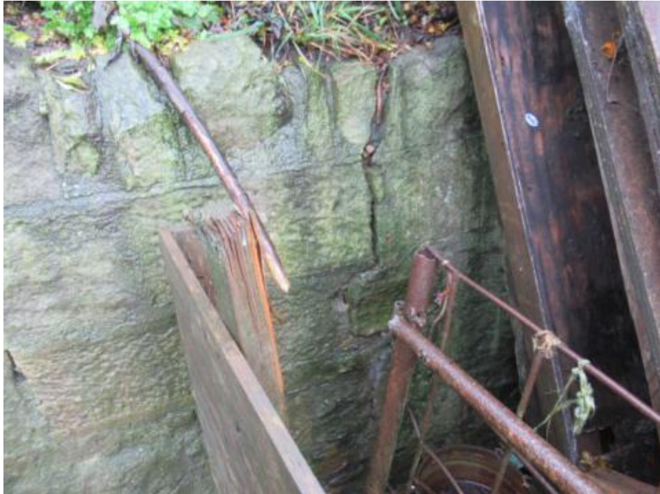
P7 – West Elevation structural cracking and outwards displacement of the stone
