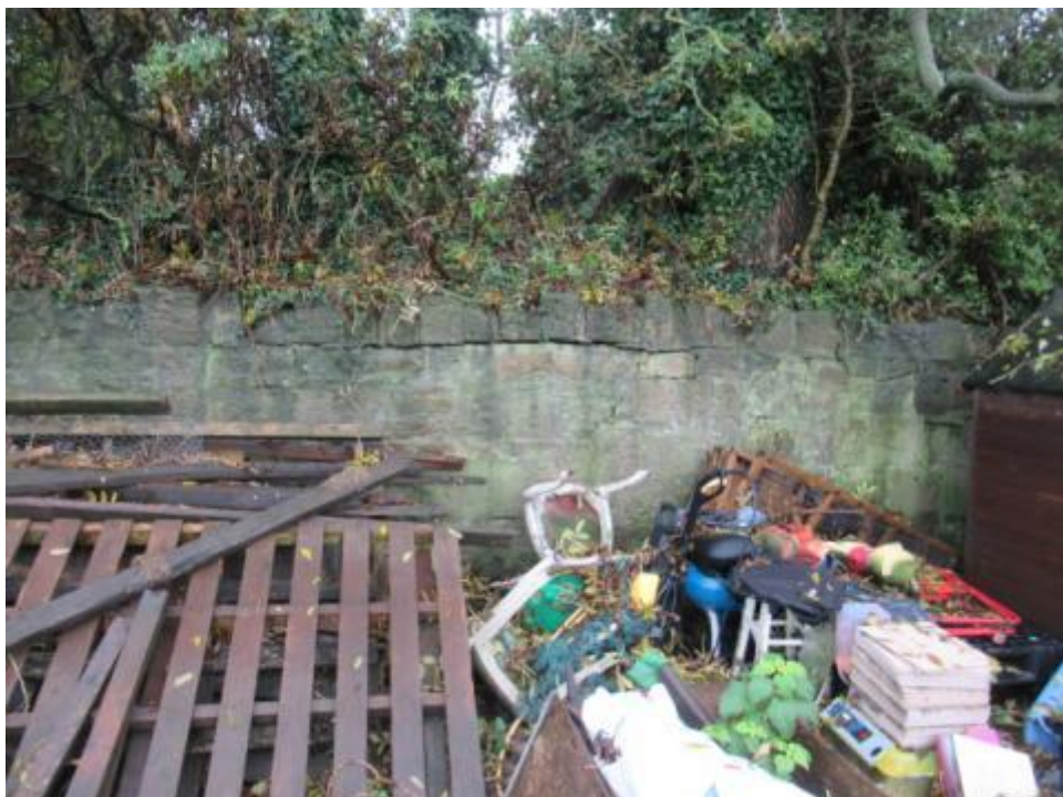
P12 – West Elevation structural cracking and displacement of the wall caused by tree root growth
