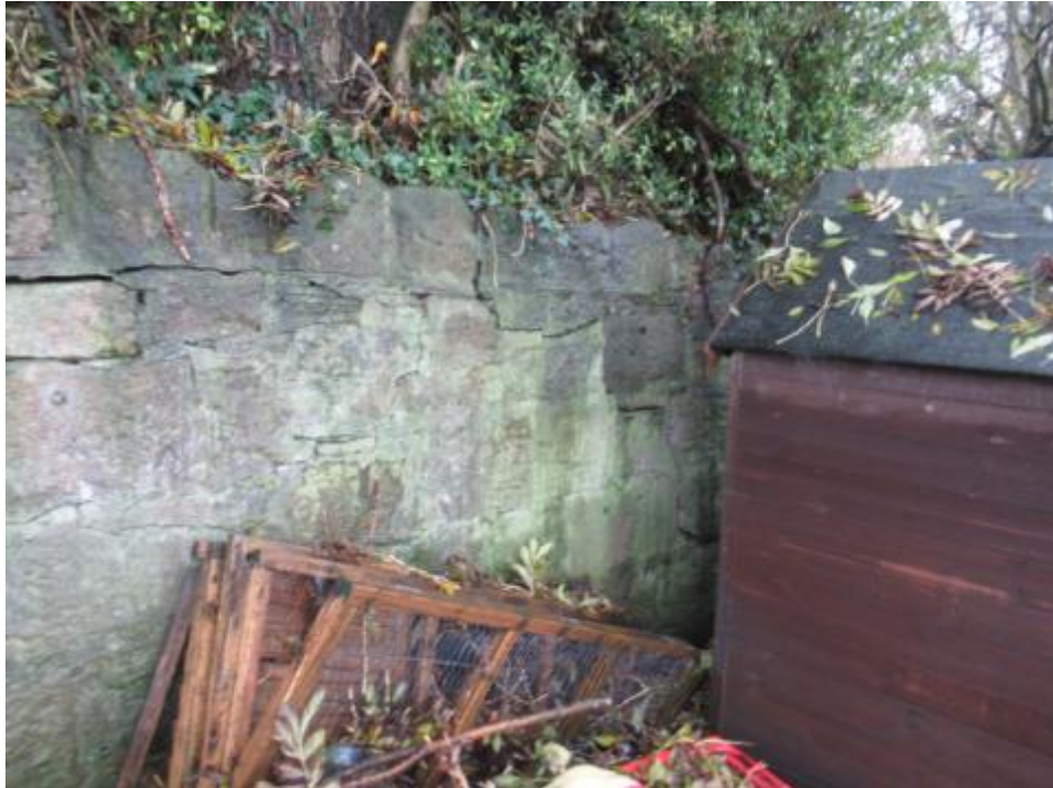
P11 – West Elevation section of structural cracking and displaced stonework to the retaining wall
