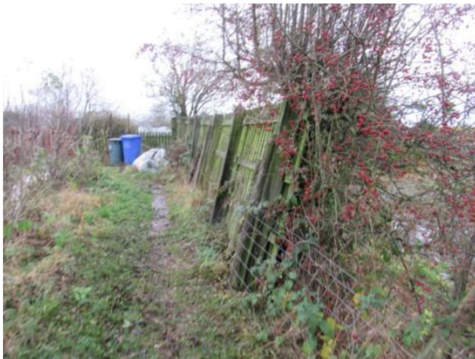
P34 – East Elevation – timber pales 4 Nr rail fence with timber posts and railway sleepers used as posts; posts collapsed and outward lean of the fence
