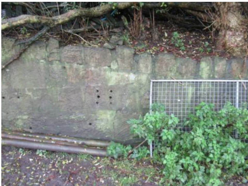
P2 - West Elevation retaining wall with reused railway sleeper blocks (holed) ( Note: structural cracking)
