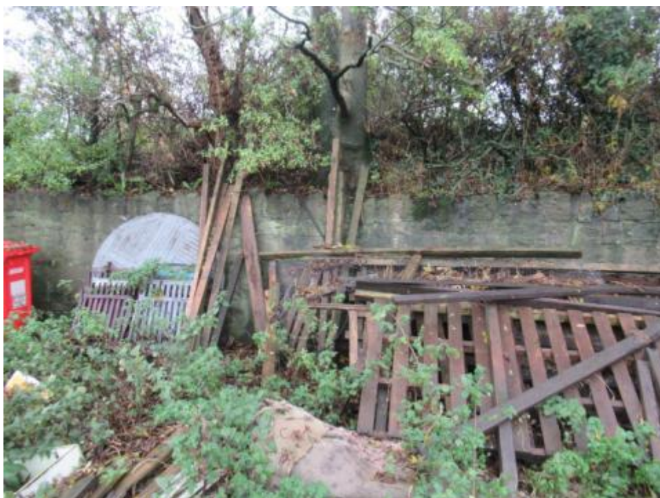
P10 - West Elevation debris stacked up against the stone retaining wall
