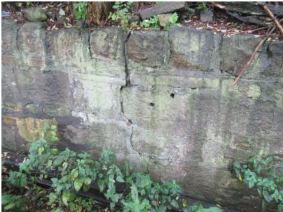
P6 – West Elevation structural cracking
