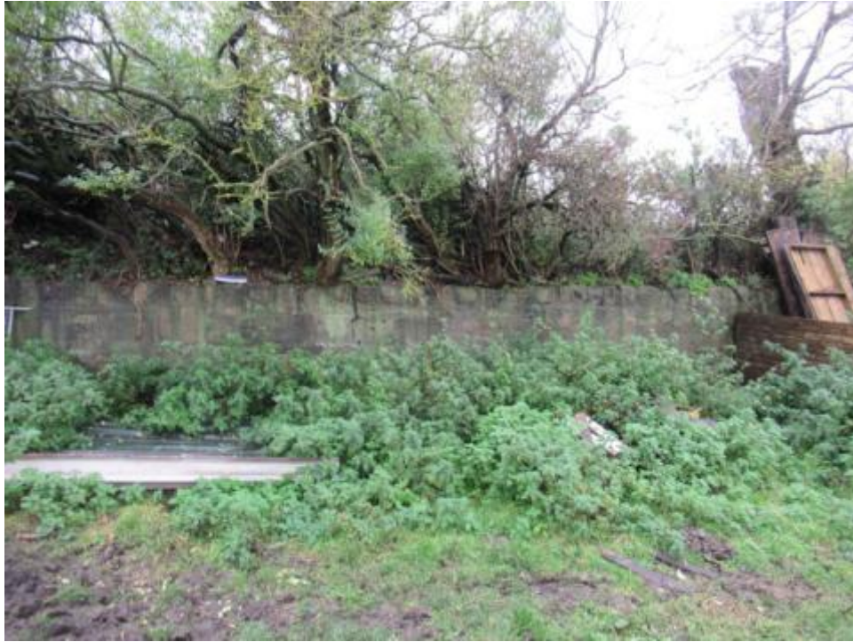
P3 - West Elevation retaining wall with reused railway sleeper blocks (holed) (Note: structural cracking over the height of the wall)
