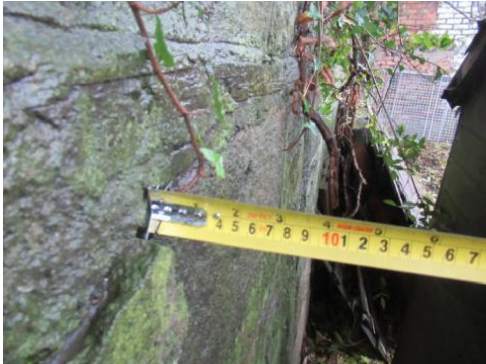
P13 – West Elevation stonework outward displacement
