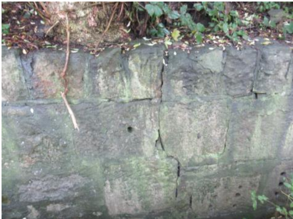
P4 - West Elevation retaining wall with reused railway sleeper blocks (holed) (Note: structural cracking)
