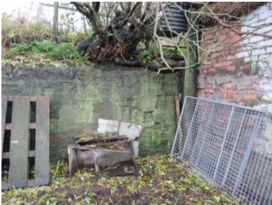
P15 – West Elevation structural cracking and displacement of the stonework adjacent to the lean-to offshot
