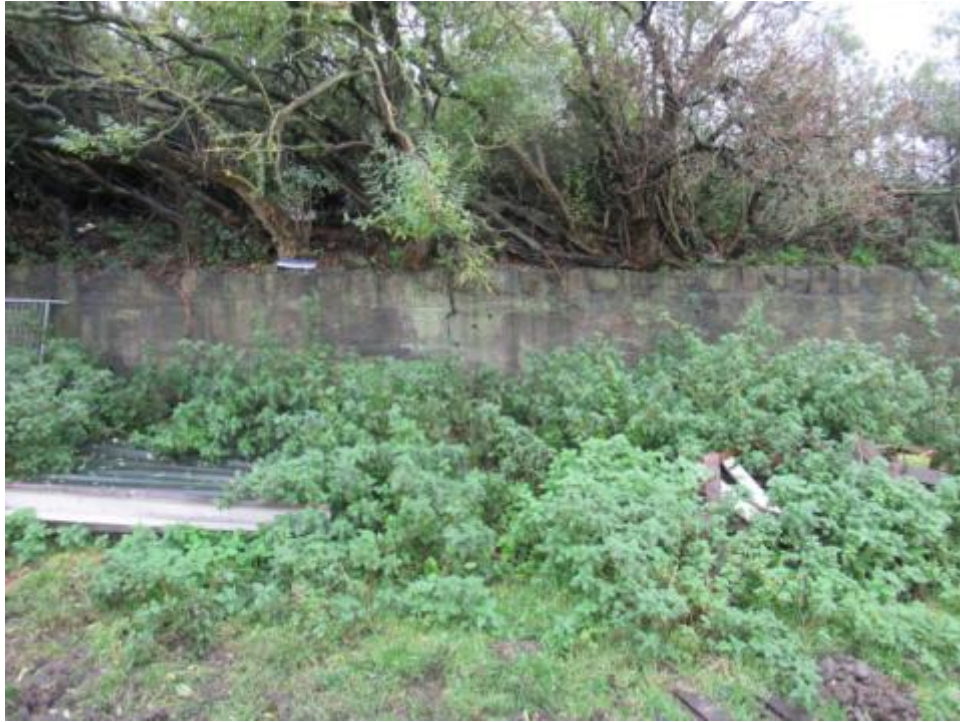
P5 - West Elevation retaining wall with reused railway sleeper stones (holed) ( Note: structural cracking)
