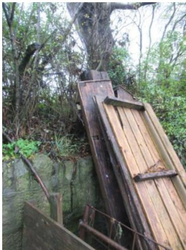
P8 - West Elevation retaining wall structural cracking and displacement indicative of outer movement
