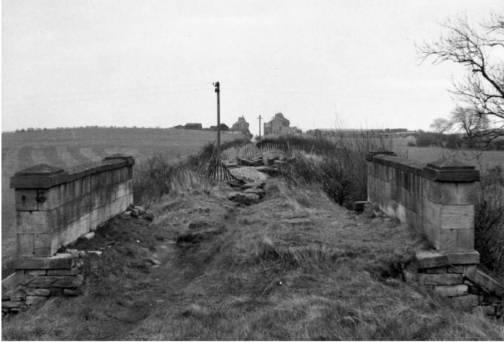
Plate 17. The decking of the accommodation arch with the road bridge decking beyond. Stone sleepers scatter the surfaces of both structures and the view of the bridge structure below the parapet shows loose stonework needing resetting and pointing. This may have been carried out in 1966, based on Vera Chapman's account (2005, 72). The photograph is undated but the parapet appears to have been removed from the road bridge. The decking stonework appears to be loose and that is still the case today. (Photo: J.W Armstrong/ Armstrong Railway Photographic Trust: 0392-3B)
