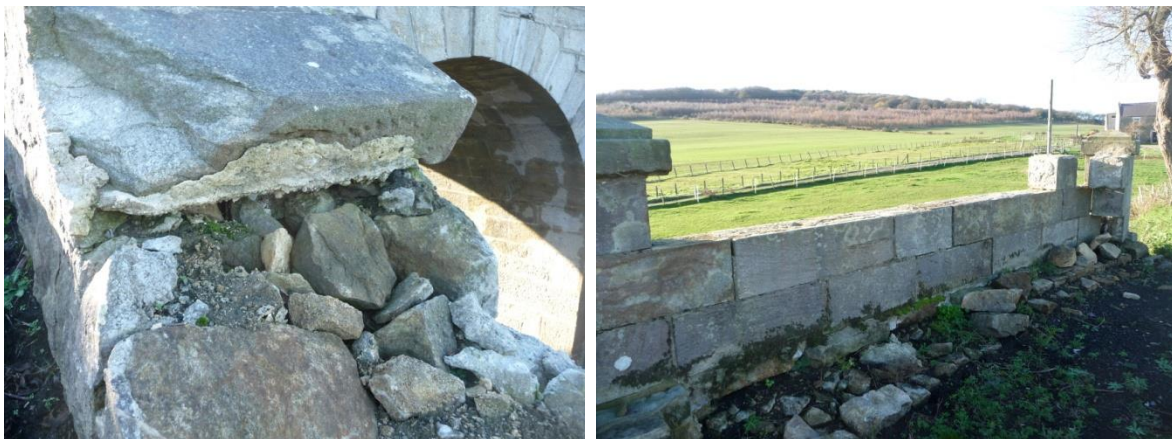
Plate 19. Left: The damaged retaining walls show that they were made of dressed stone with a rubble core and that lime mortar was used. Right: The south parapet has been partially dismantled and the west end pushed over ready to topple. The foundations of the parapets and the stone decking are also exposed.
