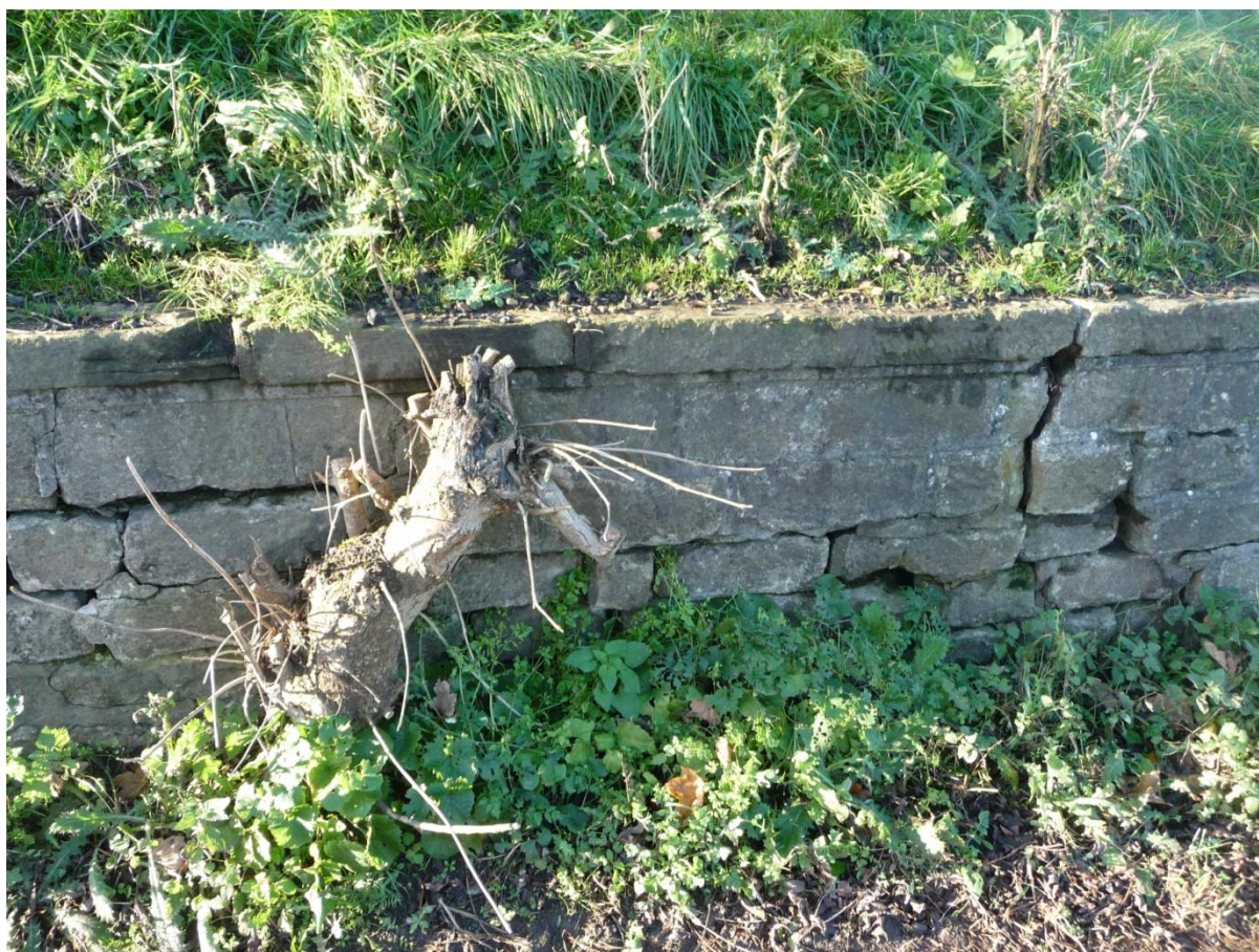
Plate 13. The retaining walls are bulging and will require consolidation. This may also be an opportunity to remove the cement render on the scarring of the original bridge.
