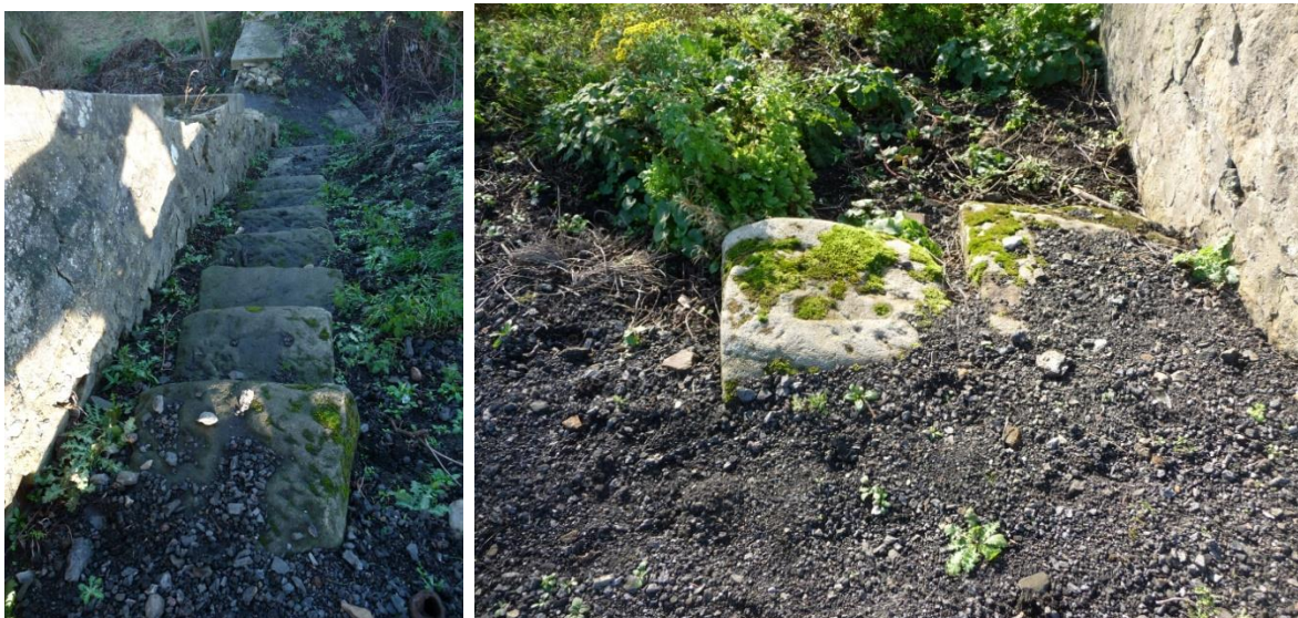
Plate 21. Left: Sleepers have been reused to form the steps from the bridge to the road. Right: Sleepers have been dislodged and are being pushed to the edge. These were originally designed to be as large as 'one man' could carry and so are vulnerable to theft.
