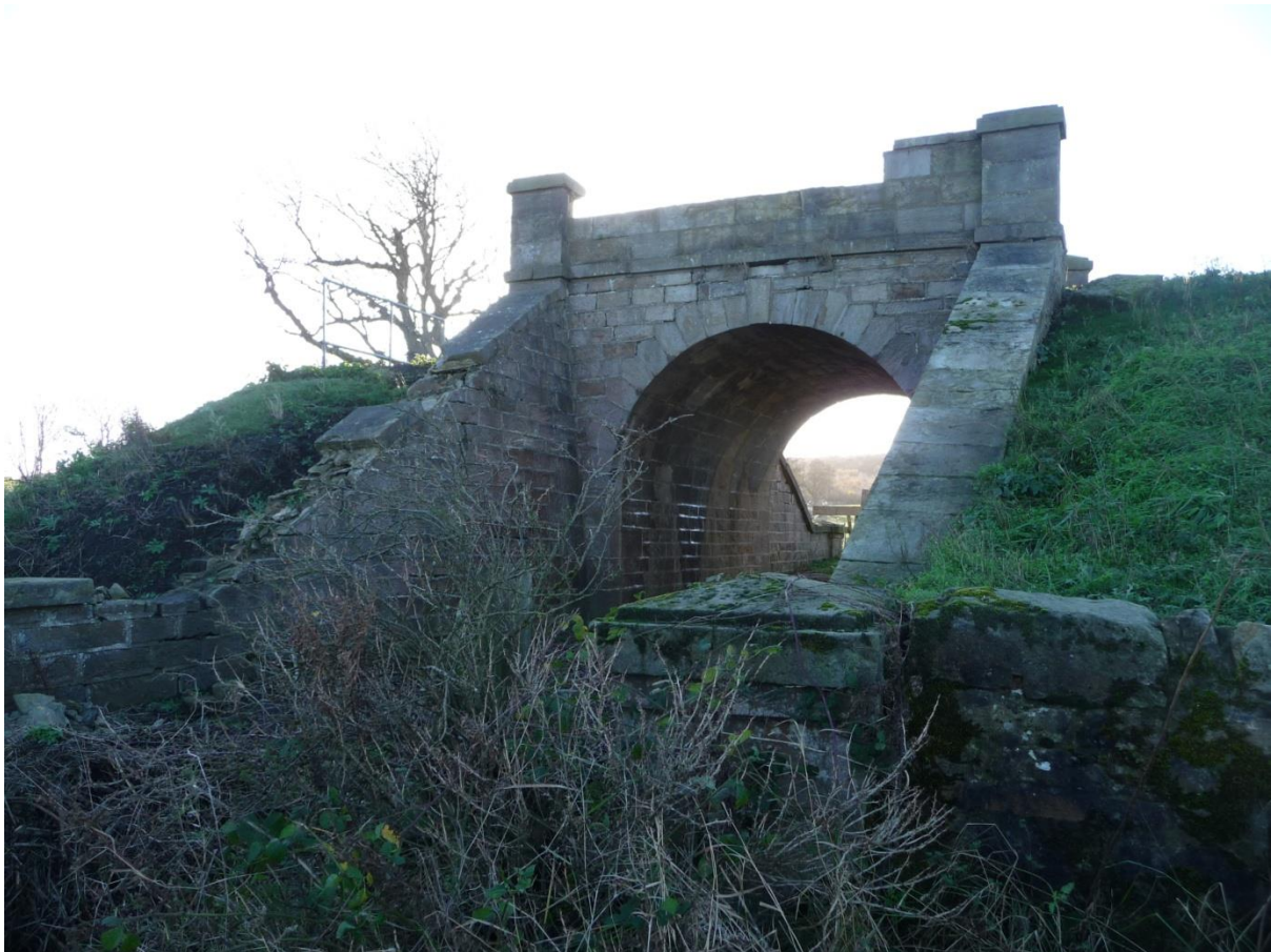
Plate 20. Part of the parapet has been dislodged and toppled while the coping stones from one of the retaining walls have been removed.
