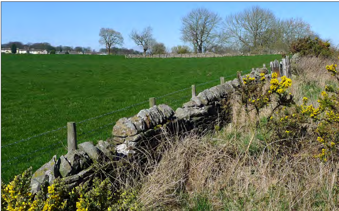
Fig 12: The original railway boundary wall to the south of the Etherley Engine. Ground inspection revealed most of the coping stones are in place. March 2019 © Historic England.
