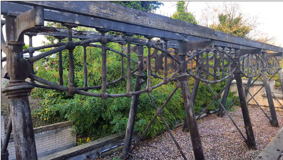
Fig 13: The bridge over the River Gaunless was the world's first iron railway bridge. It is now preserved at the National Railway Museum, York. October 2018 © Historic England.
