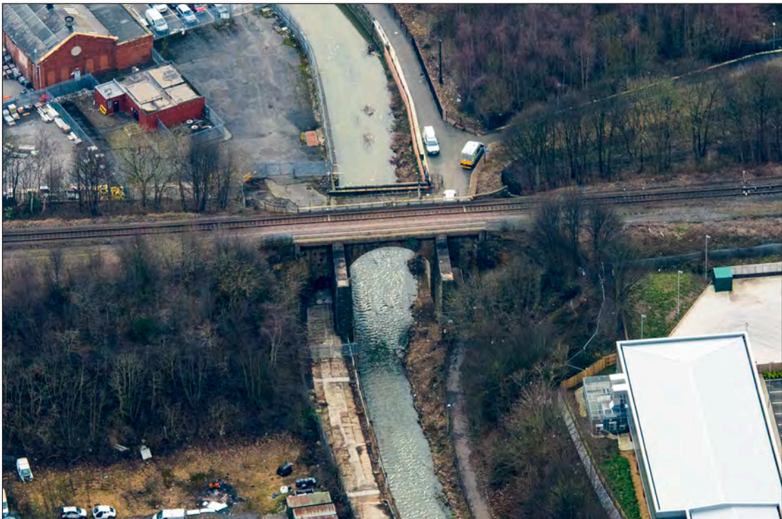
Fig 30: The north elevation of the Skerne Bridge (AIM75) shows late 19th century supports for the widening of the bridge. Detail of 28985_009 22-FEB-2018 © Historic England.
