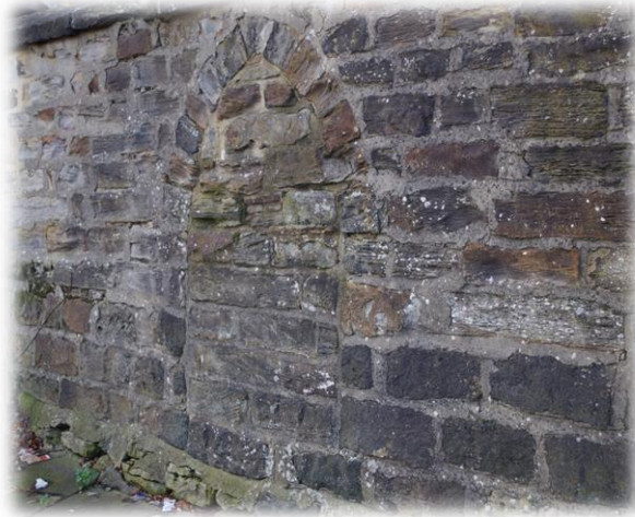
Plate 12. A blocked neo Gothic - style door in the coal depot boundary wall.
