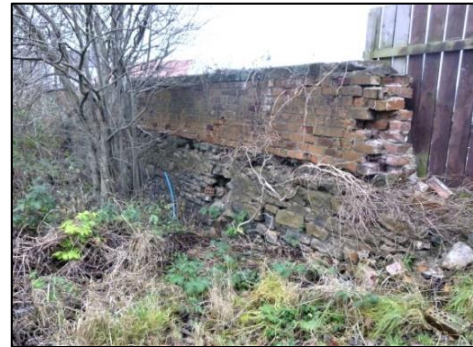
15. The retaining wall needing repair (right)
