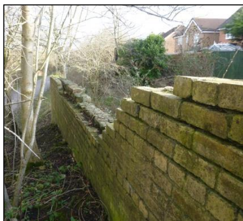
10. Old Mill wall; damaged eastern end (left).
